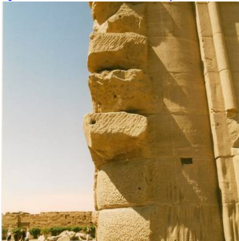
Fig. 14. Unfinished wall corner Kiosk of Trajan.
